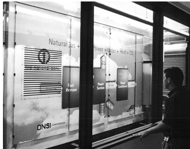
Fuel cell provides reliable digital quality power to the First National Bank of Omaha credit card processing center. Today's digital economy increasingly demands premium quality power; driving growth in distributed generation.
