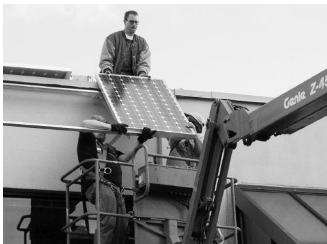
Solar photovoltaic modules installed at Puget Sound Electrical Joint Apprenticeship & Training Committee's Renton Training Center in photovoltaics training program.
